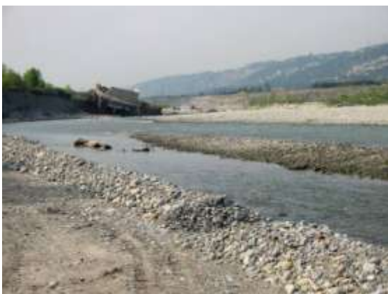
Plant 3, after destruction of sill number 3 by the 1994's flood, Var, France
