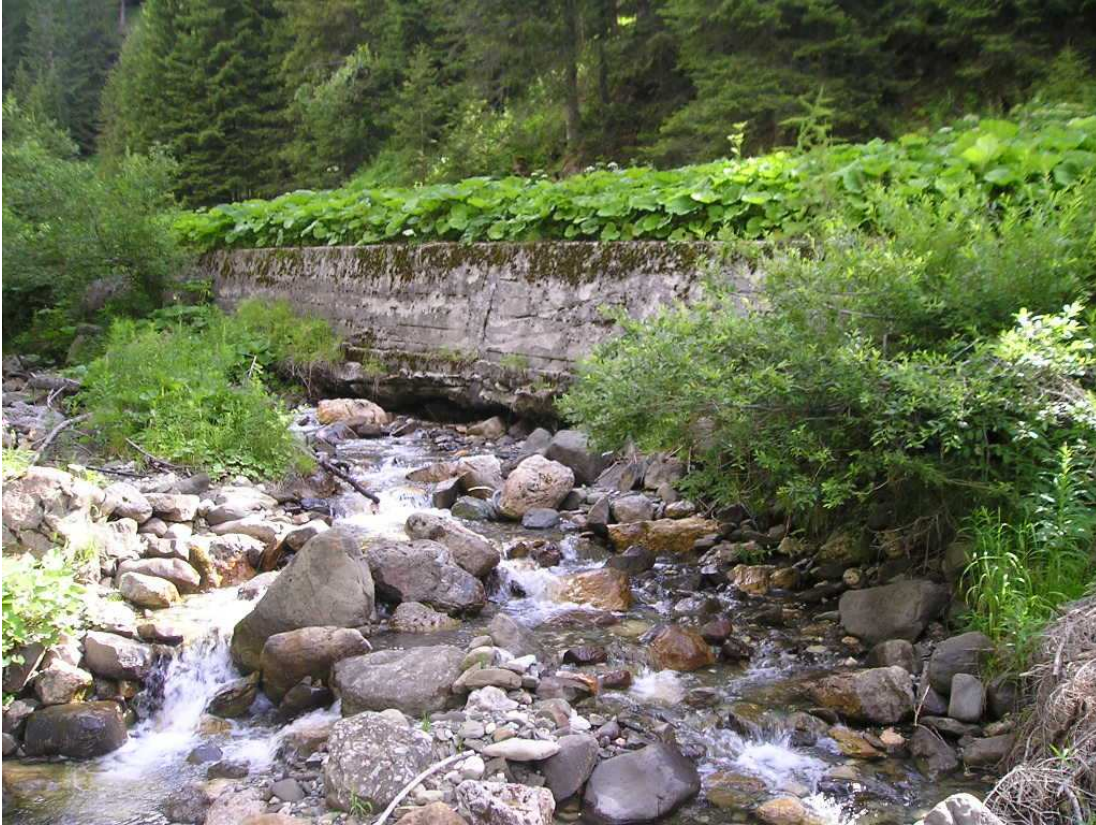
Figure 78: check dams and lateral bank protection works along the channel reach downstream the withdrawal point
