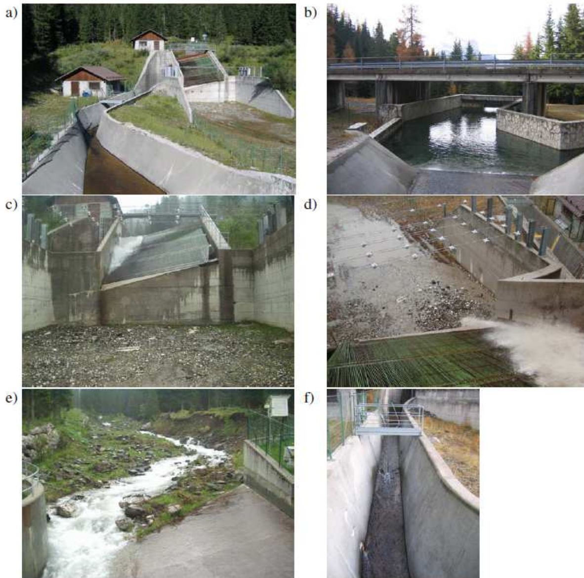
Figure 68. Rio Cordon measuring station: a) Downstream view of the bedload storage, the outlet flume and the two buildings hosting instrumentations and the emergency power system; b) Upstream view of the fine sediment settling basin; c) Downstream view of the separating grid, the bedload storage area and the cable frame which host the 24 ultrasonic sensors; d) Upstream view of the bedload storage area; e) Downstream view of the inlet channel; f) Downstream view of the outlet channel. (From Mao et al., 2010)
