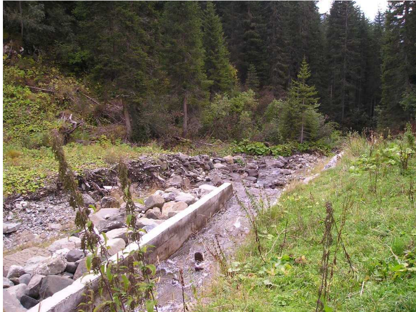
Figure 74: withdrawal point at 1639 m s.l.m.; small check dam and lateral channel for DMV ensurance
