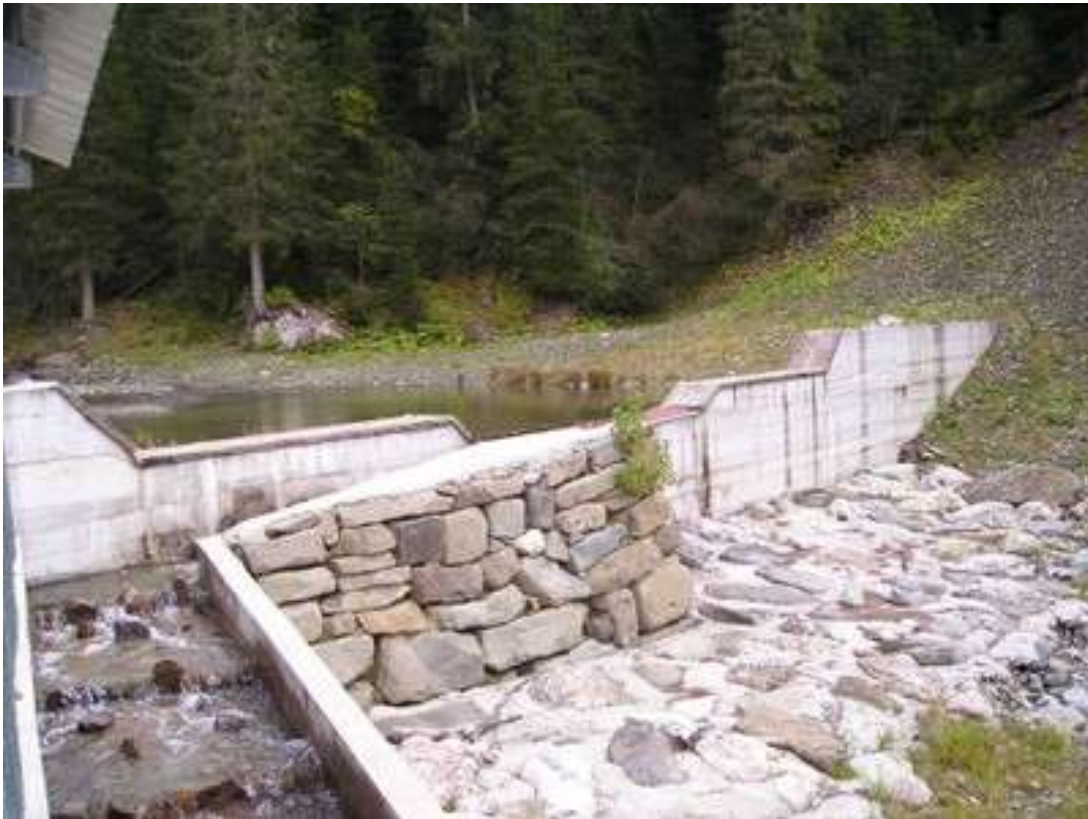
BIM HP plant intake. The water abstraction work is made of a grid placed on the top of the check dam
