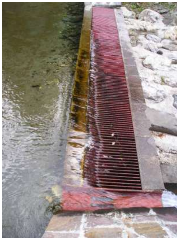
BIM HP plant intake: detail of the grid on the top of the check dam
